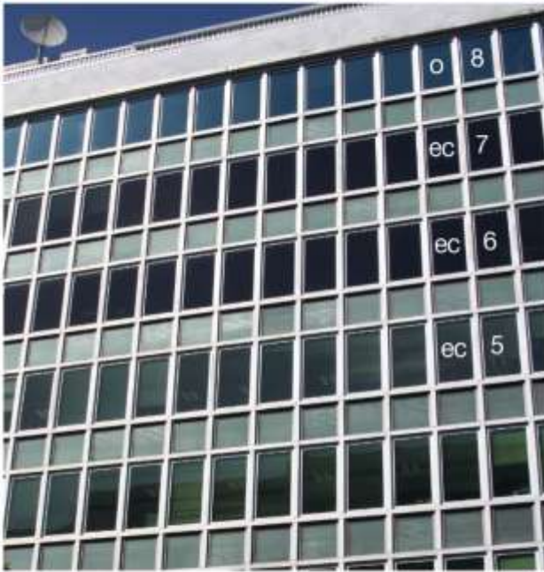
Figure 2. Outdoor view of the south façade with electrochromic (ec) and original (o) windows.
