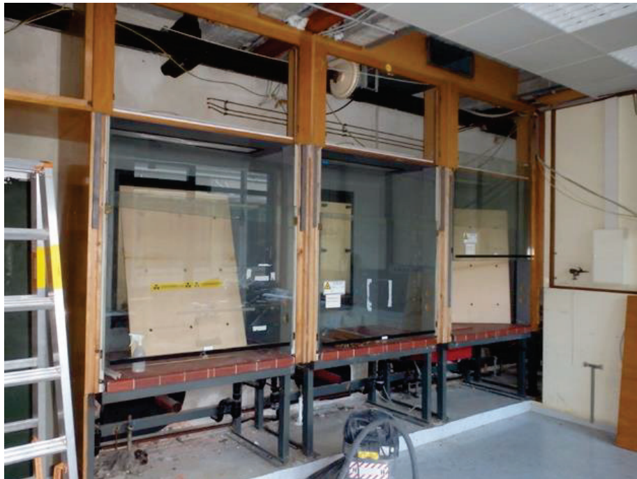
Figure D-17: Dismantling of the digestories in a radiochemical laboratory of the RCM (Copyright: Brenk Systemplanung GmbH)
