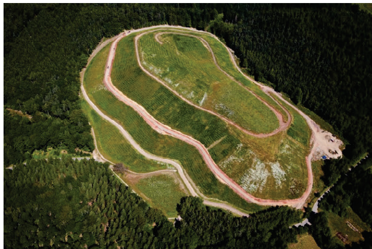
Fig. 3: Covering of heap 309 in Bad Schlema completed (as of July 2016, copyright: Archive Wismut)
