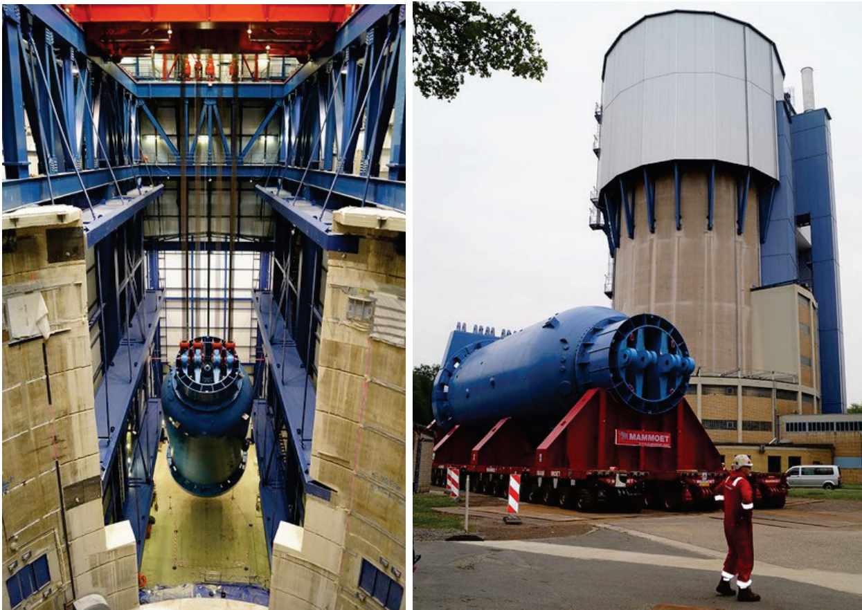
Figure D-16: Left: tilting the reactor vessel suspended on strand jacks in the material lock; right: transport of the reactor vessel to its storage facility by a heavy-duty system (Copyright: EWN)
