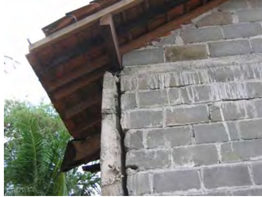
Figure 20. Insufficient connection between wall and tie column and between tie column and bond beam, Segoroyoso, Pleret (Bantul) S7.88174° E100.40869°, IMG_6749
