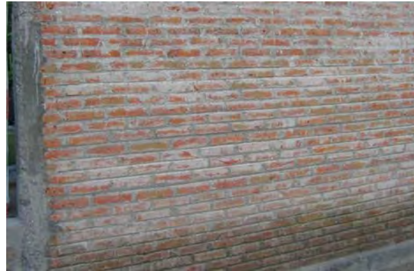
Figure 2. Well-built confined masonry wall, house on edge of heavily damaged Pleret (Bantul), S7.83686° E110.41552°, IMG_6640
