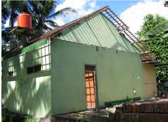
Figure 4. Masonry gable wall out-of-plane failure in 27 May 2006 Central Java Earthquake, Keputren, Pleret (Bantul) S7.86905° E110.40272°, IMG_6721
