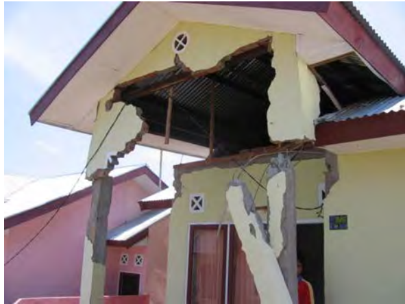
Figure 13. Subdivision of confined masonry houses, damage to covered terrace, Bengkulu. S3.83218° E102.29287
