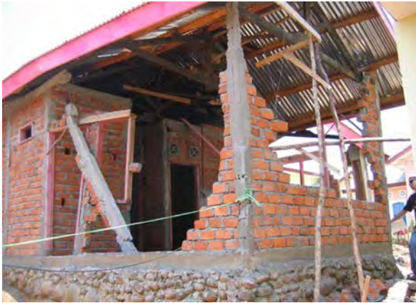
Figure 21. Subdivision of confined masonry houses, collapse of masonry wall exacerbated by insufficient connections, Bengkulu. S3.83218° E102.29287
