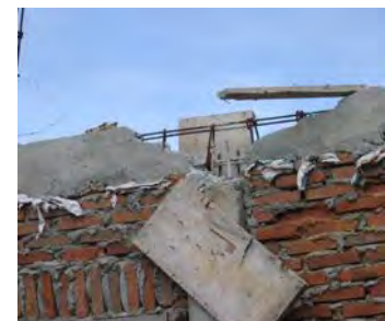
Figure 14. Bad practice, connections and concrete quality, other organizations
