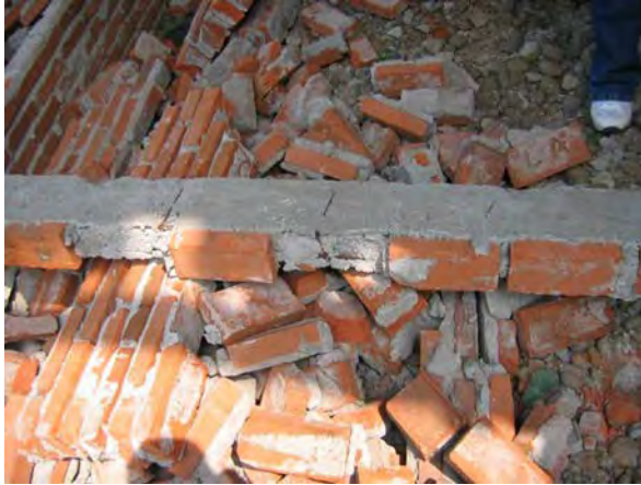
Figure 23. Close up view of collapsed ring beam and wall, same as Fig. 20. Failure plane between top of mortar bed and bottom of brick above it.
