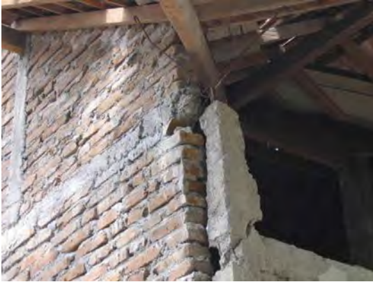
Figure 19. Insufficient connection between wall and tie column and between tie column and bond beam, Pleret (Bantul) S7.88174° E100.40869°, IMG_6746
