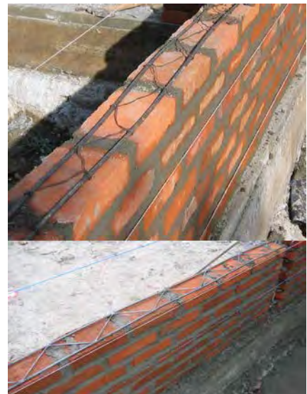
Figure 9. Horizontal reinforcement fabricated on-site with binding wire (top) and prefabricated at welding shop (bottom).
