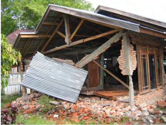
Figure 8. Collapse of front wall in confined masonry house , Padang Panjang, IMG_8831
