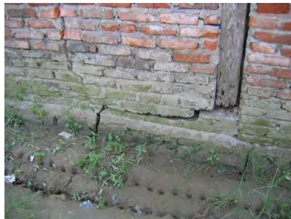
Figure 26. Cracks in foundation and walls associated with settlement and tilt on liquefiable soils, Lempuing (Bengkulu), S3.82799° E102.28473
