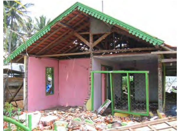
Figure 9. Partially collapsed brick masonry house with reinforced concrete (RC) tie columns and timber bond beams, note partial collapse of masonry gable wall, and lack of in-plane stiffness in front wall, Kec. Lais (North Bengkulu) S3.53217° E102.03771
