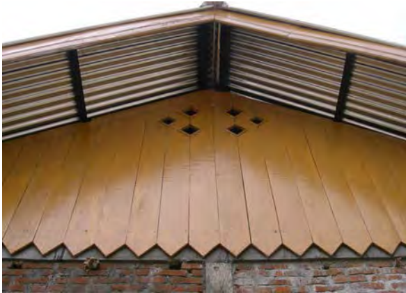
Figure 6. Papan Gable (Maimunah's house designed and built by Build Change, Keunue ue, Peukan Bada, Aceh Besar)
