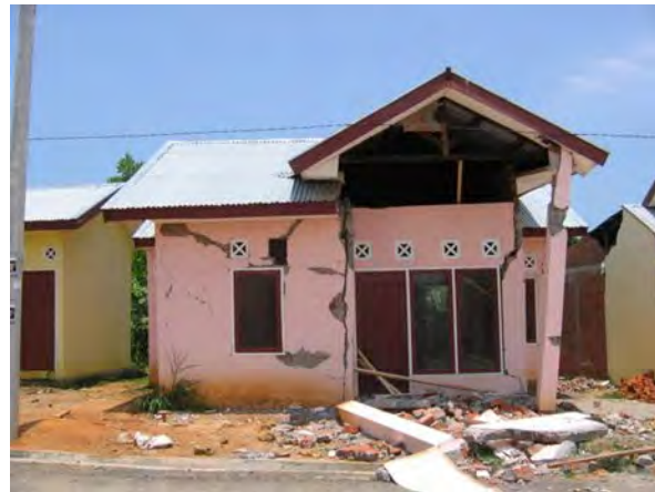
Figure 14. Subdivision of confined masonry houses, damage to covered terrace, Bengkulu. S3.83218° E102.29287
