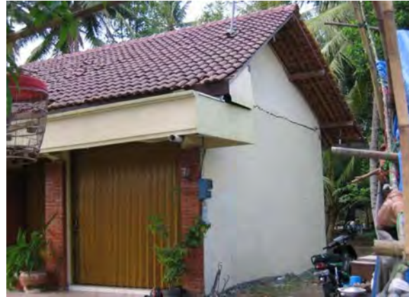
Figure 5. Masonry gable wall out-of-plane failure in 27 May 2006 Central Java Earthquake, (Bantul) S7.89468°, E110.37341°, IMG_6542
