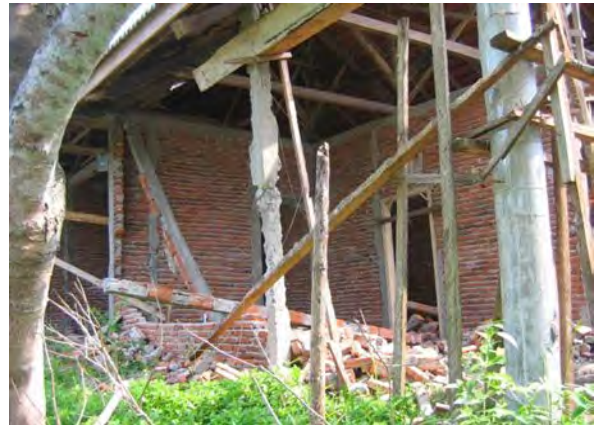
Figure 22. Confined masonry house with failure in masonry walls and connections between tie columns and bond beams, Kec. Airnapal (North Bengkulu)
