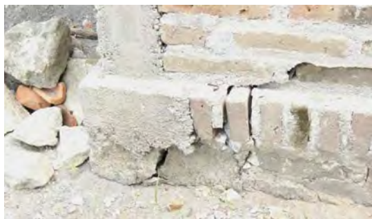
Figure 25. Displacement along wall/foundation interface, Tegal Kebong Agung, Imogir (Bantul) S7.93434° E110.36667°, CIMG1769
