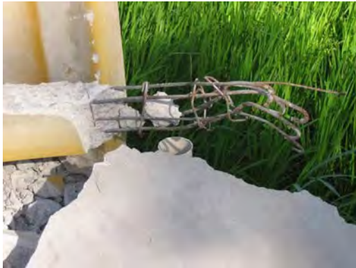
Figure 18. Connection failure, RC frame building, Central Java
