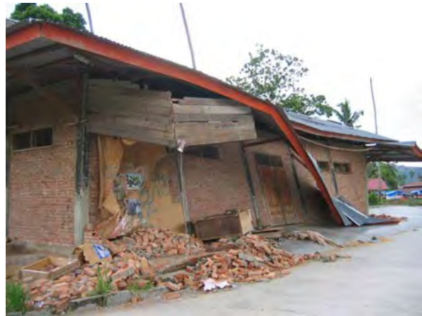
Figure 12. Confined masonry warehouse with out-of-plane failure of long walls without cross-bracing, , IMG 8891
