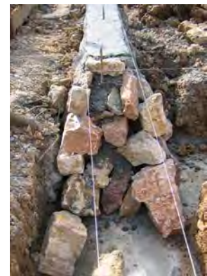
Figure 11. Poorly built stone masonry foundation. Note gaps between stones, stones standing on end.
