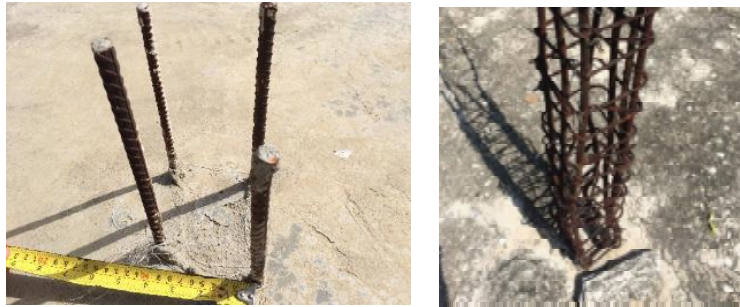
Fig. 7 – Left – Existing column extension with (3) #4 and (1) #3 bars Right – Existing column extension with smooth rebar and stirrups already placed
