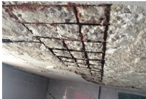
Fig. 8 - Existing slab in poor condition
