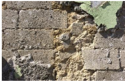
Fig. 6 – Poorly repaired wall crack
