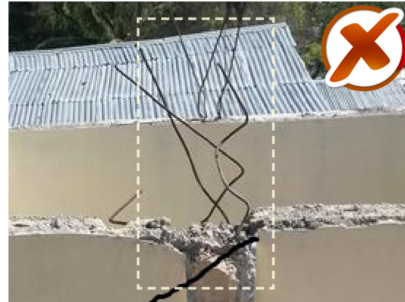
2. Extensions that are significantly bent or corroded or are less than 60cm long should not be used to connect the expansion to the existing building below and will need to be replaced.
