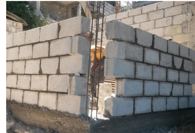
1 – Build the wall up to the level of the existing intermediate ring beam, or up to 1m20 if there is not an intermediate ring beam in the adjacent existing wall. Refer to the Retrofit Practical Handbook 1 page 16 “Wall Construction” for more details.
