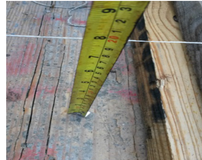
14. Use string lines to define the thickness of the slab (minimum 20cm, total for a alveol slab, including the 5cm concrete topping).
