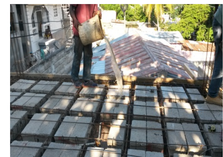
15. Wet the formwork and the blocks to improve the concrete prior to pouring the concrete.
