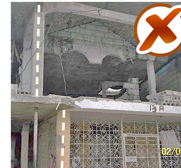
All columns should be aligned continuous from the foundation up to the top floor.
