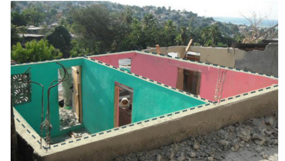
2. Prepare a clear level and regular surface on top of the blocks in order to place the new horizontal ring beam.
