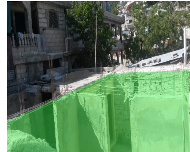
3. Demolish the existing slab or lightweight roof, particularly in areas where columns will be extended up to the vertical expansion.
