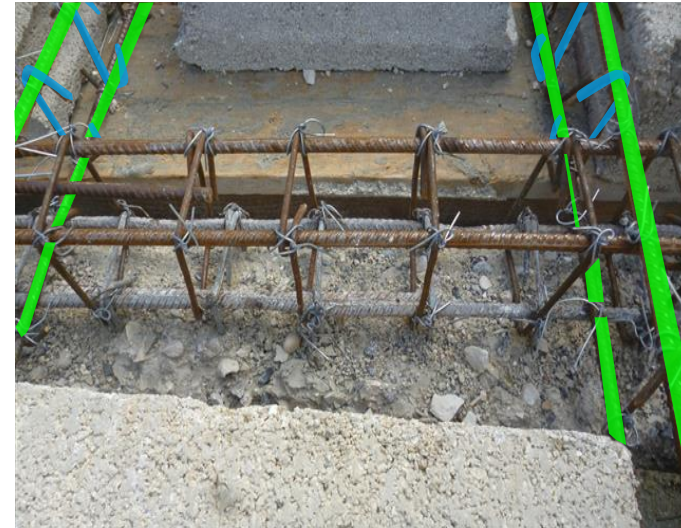
4. Considering the 4 upper rebars like a new ring beam, anchor the slab beams. Refer to the previous step by step explanation, "Construction of a New Slab" for how to finish installing the new slab.
