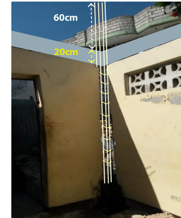
4. Where new columns at the lower level are required, install them with correct extensions above the future slab. The extensions shall be 60cm minimum from the top of the future concrete slab to the top of the vertical rebar to allow for adequate bar lap. Refer to the Retrofit Practical Handbook 1 , page 39, for detailed steps on installing a "New Tie Column in an Existing Wall".
