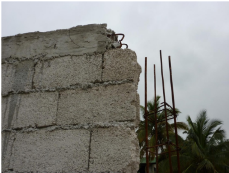
Visible rebar tree is very short
