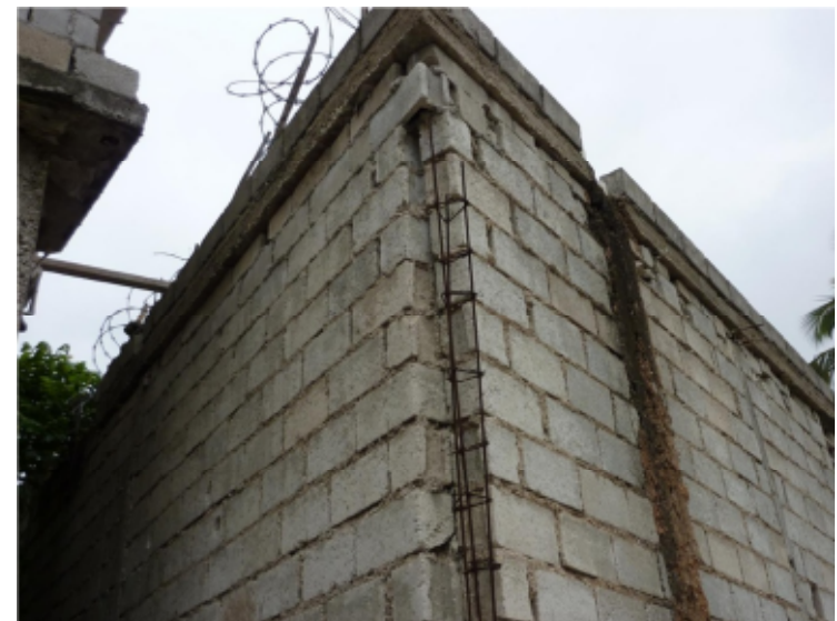
Ongoing construction reveals poor detailing
