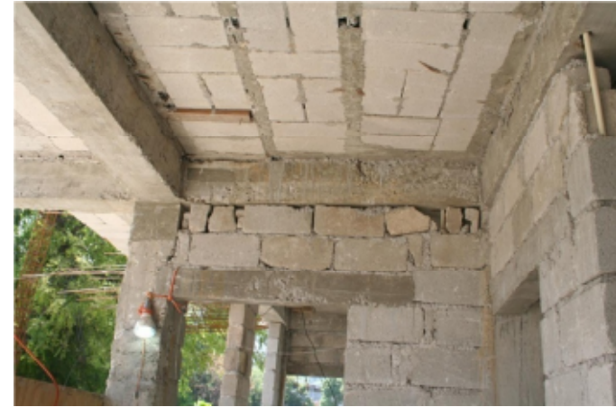
Top row of masonry not in full contact with slab or ring beam
