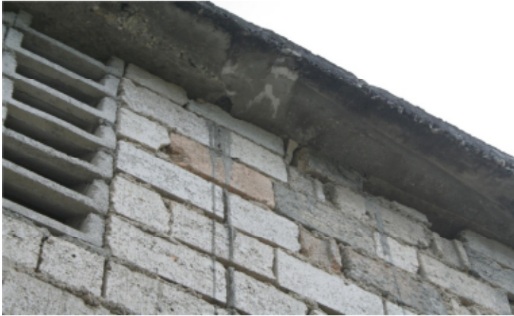
Incomplete mortar infill or no mortar in head joists, loose window infill.
