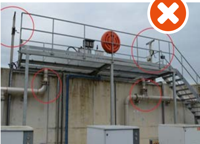
Image 9.4 Several examples of davits outside edge protection system and hand actuated valves placed at height
