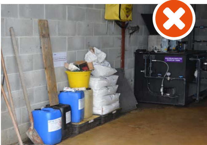
Image 6.1 Example of no design provision being made for chemical storage used in process
