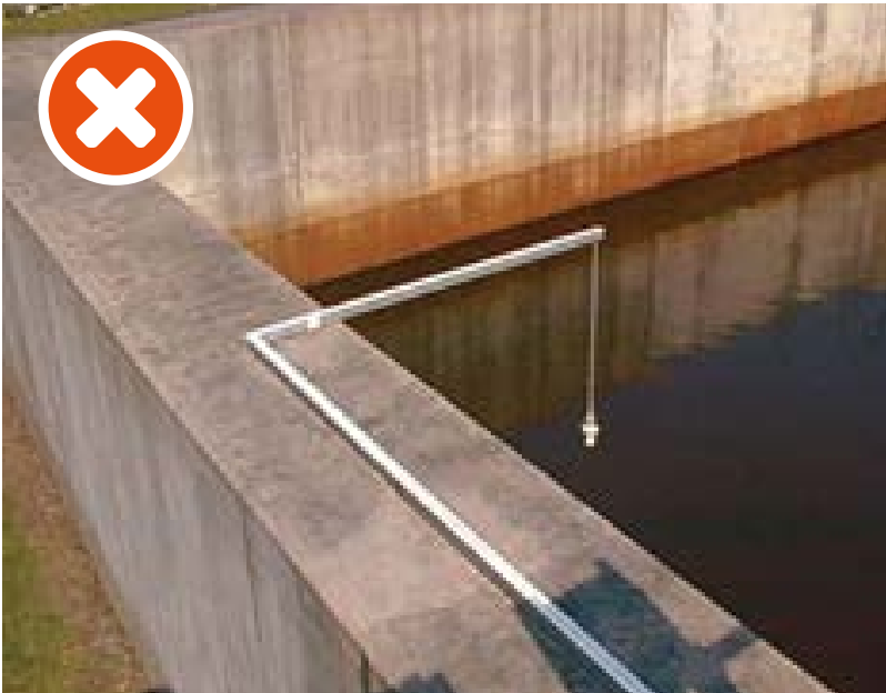
Image 1.1 The sensor is installed at height but is not easily retractable for maintenance, leading to risk of falls from height when leaning in to work on the sensor.
