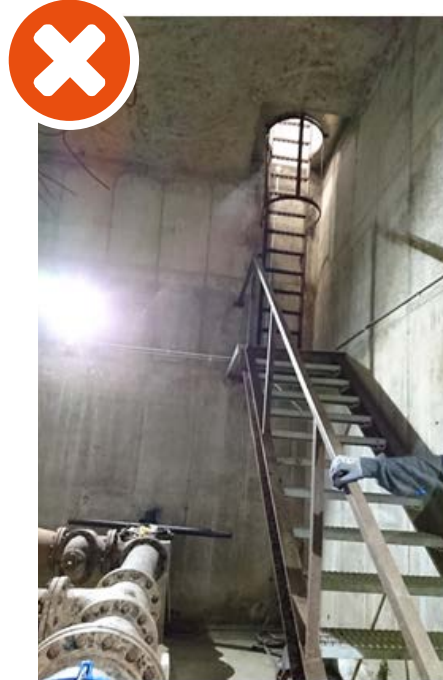
Image 5.3 Access to confined space includes ladder access. A better solution would be if the confined space was fully accessible by stairs to enhance access for emergency recovery.
