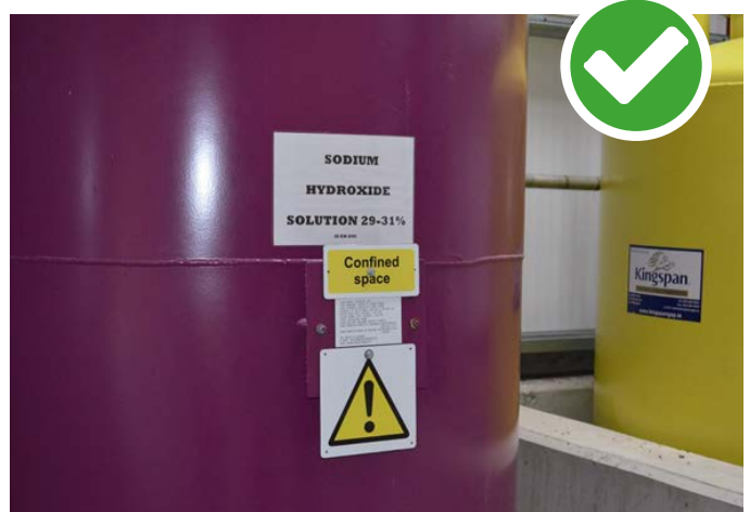
Image 6.2 Example of good provision of information and labelling with regard to chemicals
